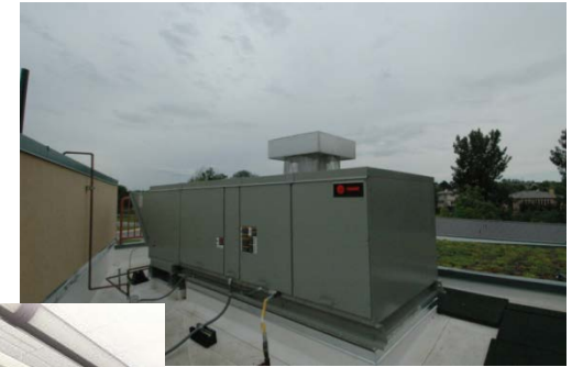
High Efficiency HVAC
